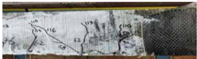
Figure 11 Crack pattern in SPB X2
