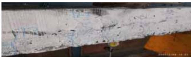
Figure 8 Crack pattern in CB-1
