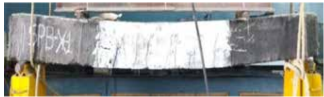
Figure 10 Crack pattern in SPB X1
