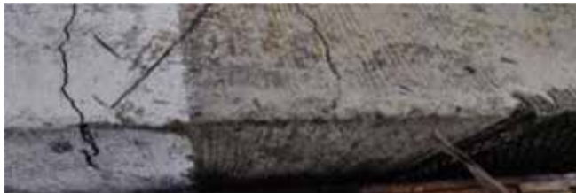
Figure 14 Shear crack occurred inside the wrapping
