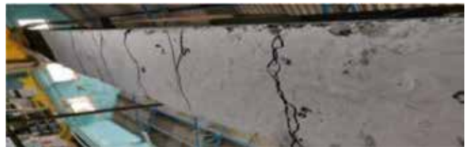
Figure 17 X2 failure mode
